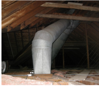
The attic holds massive air ducts which were essential to the natural aeration of the classrooms. Air flowed up and down from the cupola.
