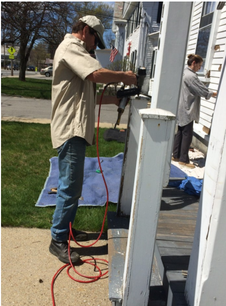
Mark and Whitney Friberg worked on the outside of the house, prepping it for painting.
